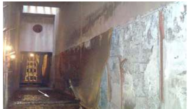
Figure 2. Damages in Sefidroud dam
