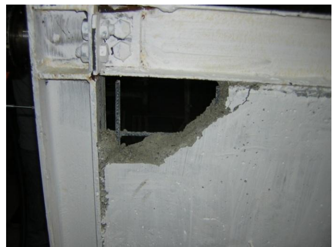
Figure 9. Complete depletion of the infill corner
