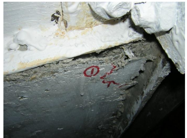
Figure 8. Concrete peeling in the corner of the infill
