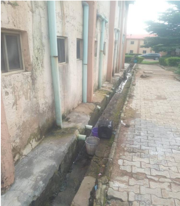
Figure 1. Grey water collection from drainage pipes in Adeniyi hostel, FUTA.
